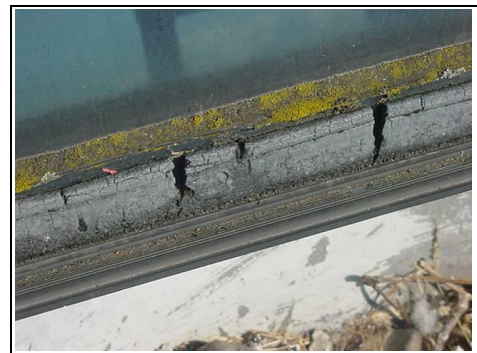
Cracks in the mastic
